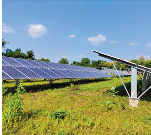
Plant A, Indra Solar Farm, Agrivoltaics plant, Tikamgarh, Madhya Pradesh. © Khare Energy Private
