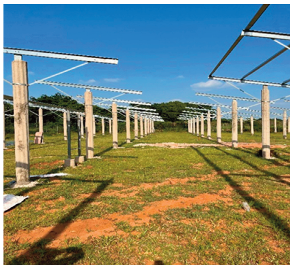
Phase 2, Indra Solar Farm, Agrivoltaics plant, Tikamgarh, Madhya Pradesh. © Khare Energy Private
