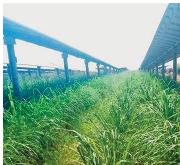
Mahindra Susten plant at Tandur with lemon grass. © Mahindra Susten.
