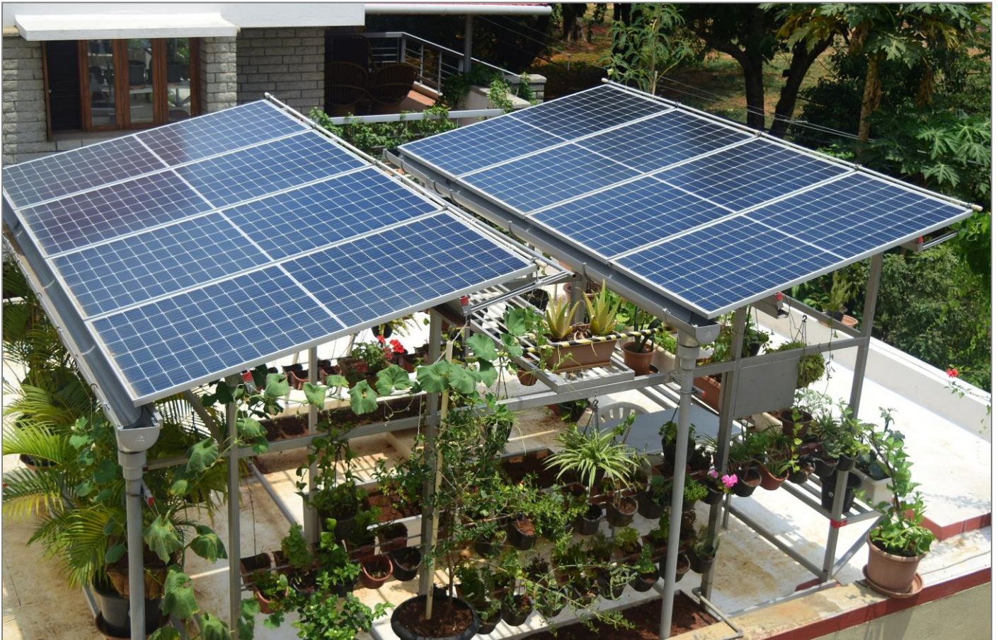
Figure 42: Hinren Agri-PV rooftop system (Credit: Hinren Engineering Pvt. Ltd.)
