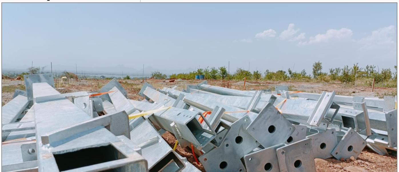
Figure 54: In the front, columns that will soon be mounted during the construction of the agrivoltaics plant near Nashik (Credit: GIZ)
