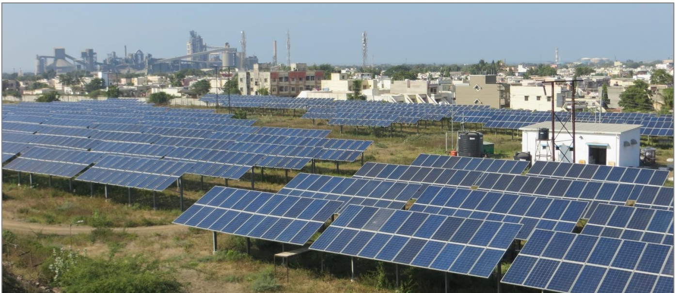
Figure 6: Harsha Abakus 1MW Sikka plant (Credit: NSEFI)
