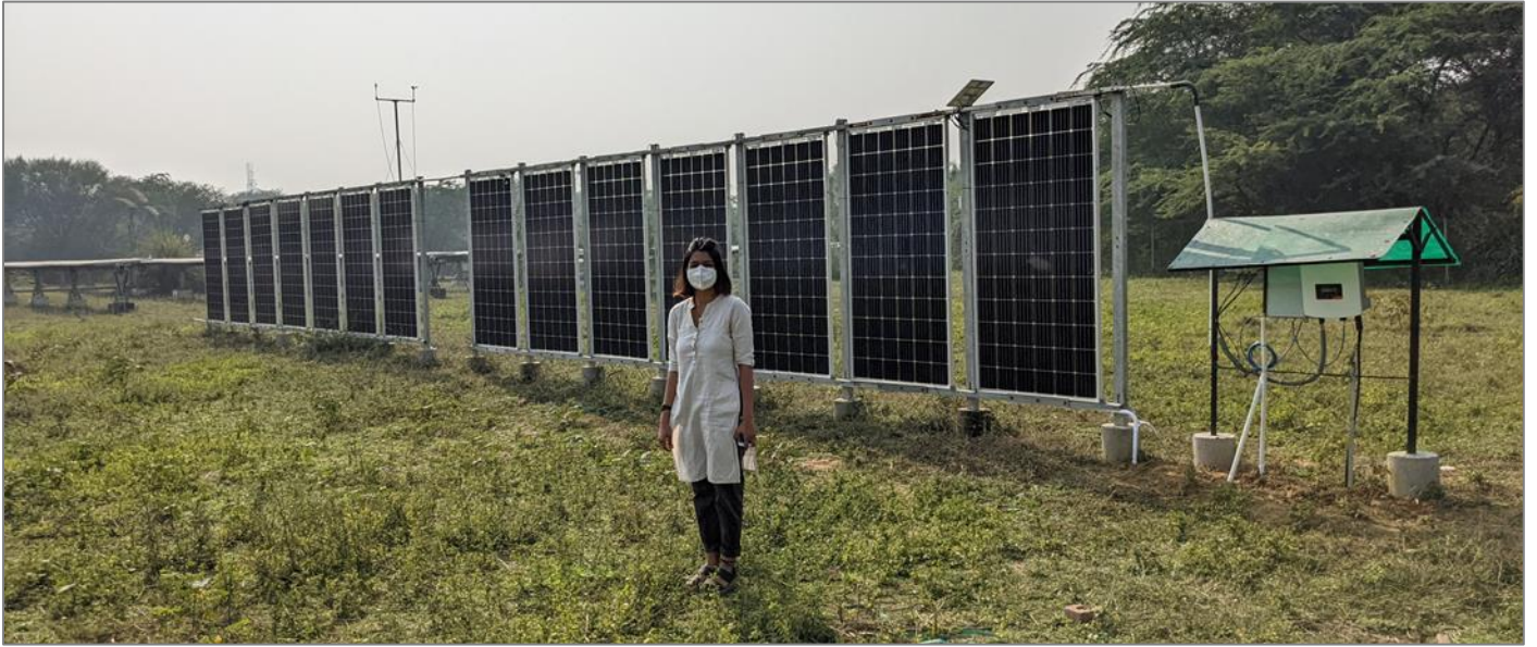
Figure 30: Vertical PV installation with bifacial modules at NISE (Credit: NSEFI)
