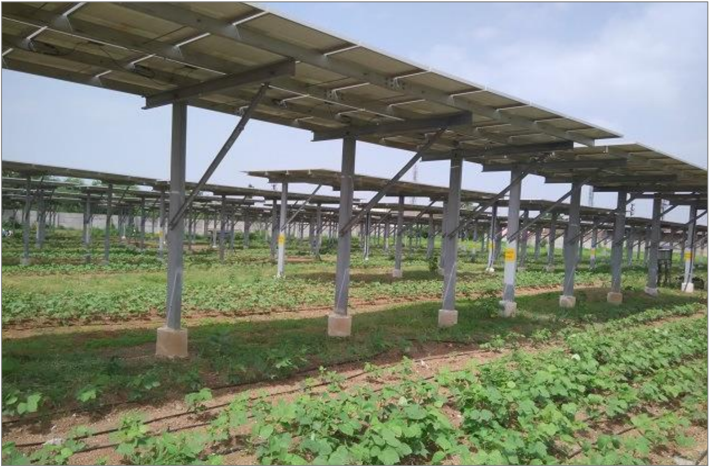
Figure 7: Harsha Abakus 1MW Panandharo plant (Credit: Hasha Abakus)
