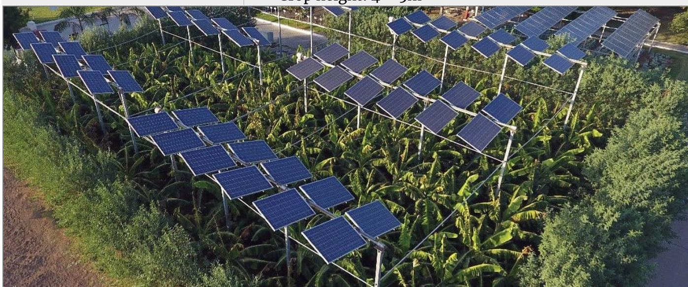
Figure 23: 14.4 kW agrivoltaic structure with banana (Credit: Jain Irrigation)
