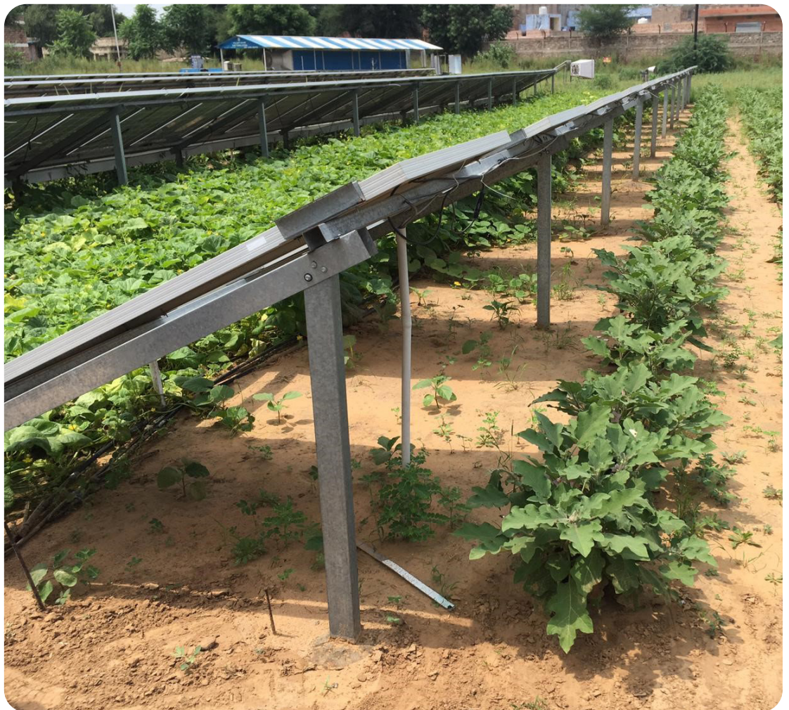
Figure 16: Chilli, 105 kW, Ground-Mounted Agrivoltaics System (Non-Elevated Agrivoltaics System/Conventional Solar), Rajasthan
