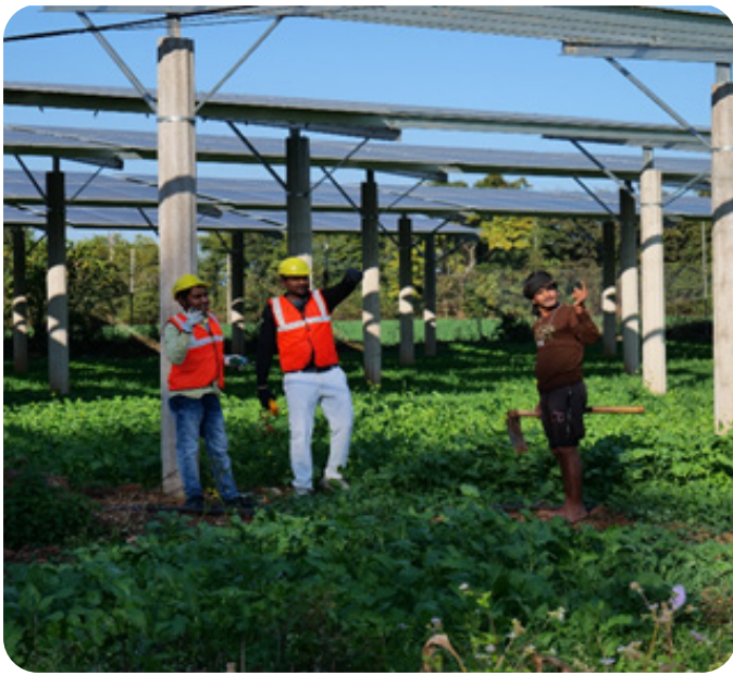
Figure 25: Operations and Maintenance of Agrivoltaics Site
