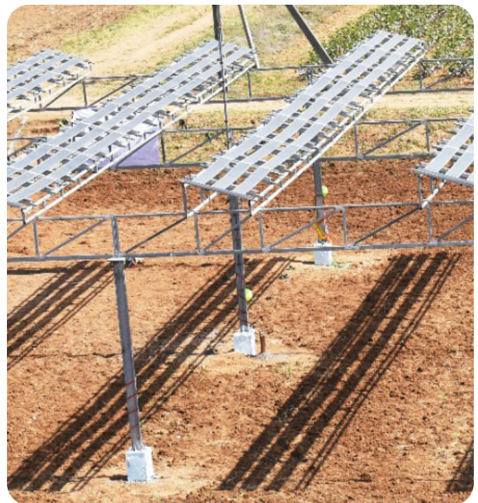
Figure 15: 10 Kw, Renkubé Agrivoltaics site in Karnataka
