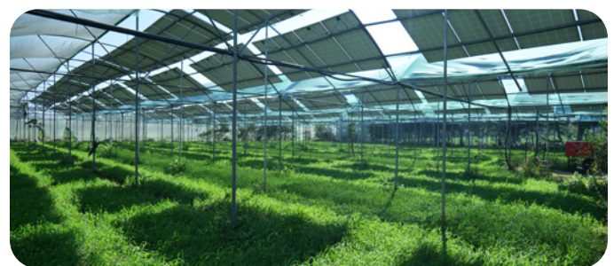
Figure 22: 1.2 MW, Greenhouse Agrivoltaics System installed by Khare Energy in Madhya Pradesh
